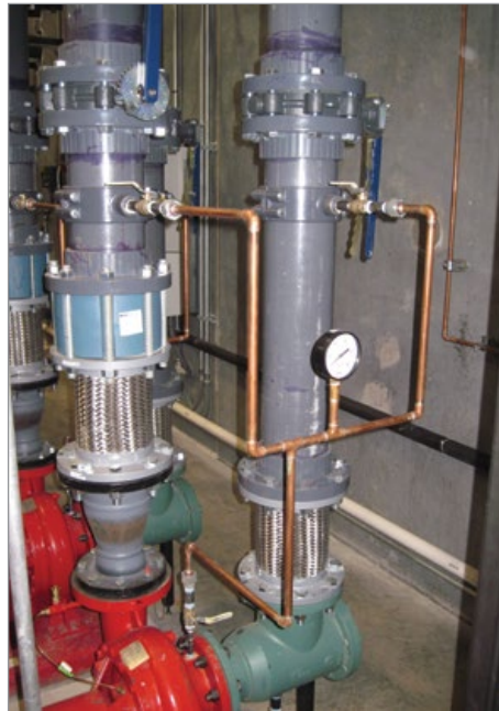
Pump pressures manifolded to a single gauge.
