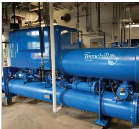
A Tecogen STx Chiller installation.
