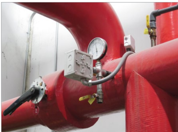
Pressure sensors showing both manual and solenoid operated blowdowns.
