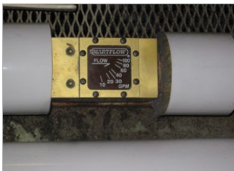
Cooling water differential pressure sensor and inline flow meters add greater depth to typical instrumentation
